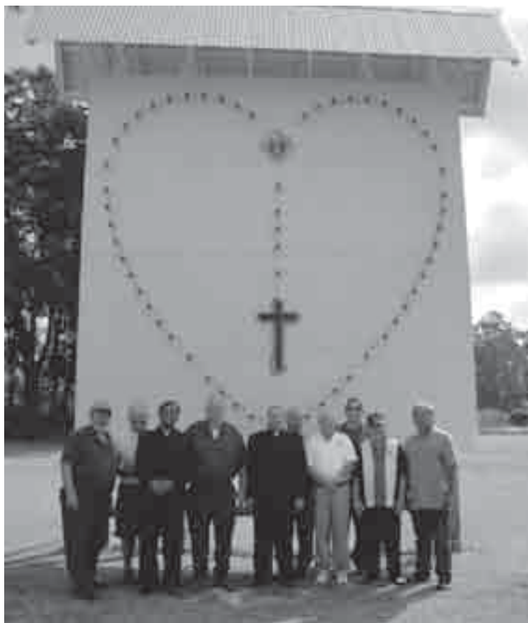
ROOF ADDED TO THE ILLUMINATED ROSARY IN MARKSVILLE. Father Rusty Rabalais, pastor of St. Joseph Church in Marksville, stands with members of KC Council #1217 who recently added a roof over the Illuminated Rosary in Marksville. The rosary will be prayed around the illuminated outdoor rosary every Thursday night from May through October.
